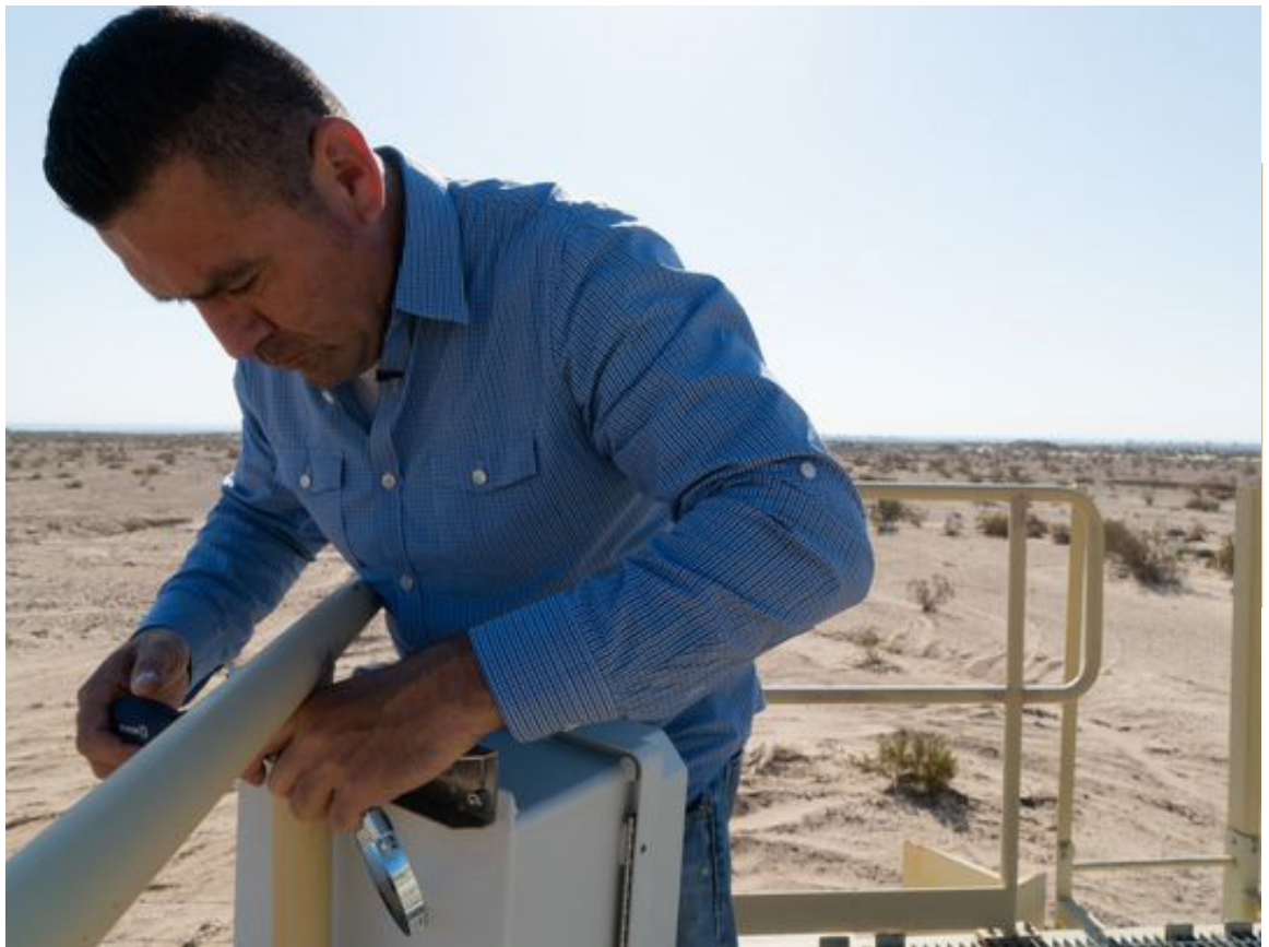
Humberto Lugo of Comite Civico del Valle installs a monitor near the Salton Sea. Each monitor installation is unique and may require different tool or materials. Photo courtesy of Zoe Meyers/The Desert Sun.
