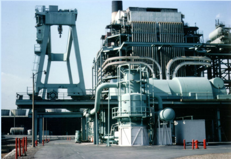
Etiwanda Generating Plant SCE, Mohave Desert 1982
