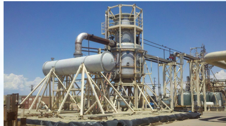
CalEnergy Geothermal Plant, Salton Sea 2022
